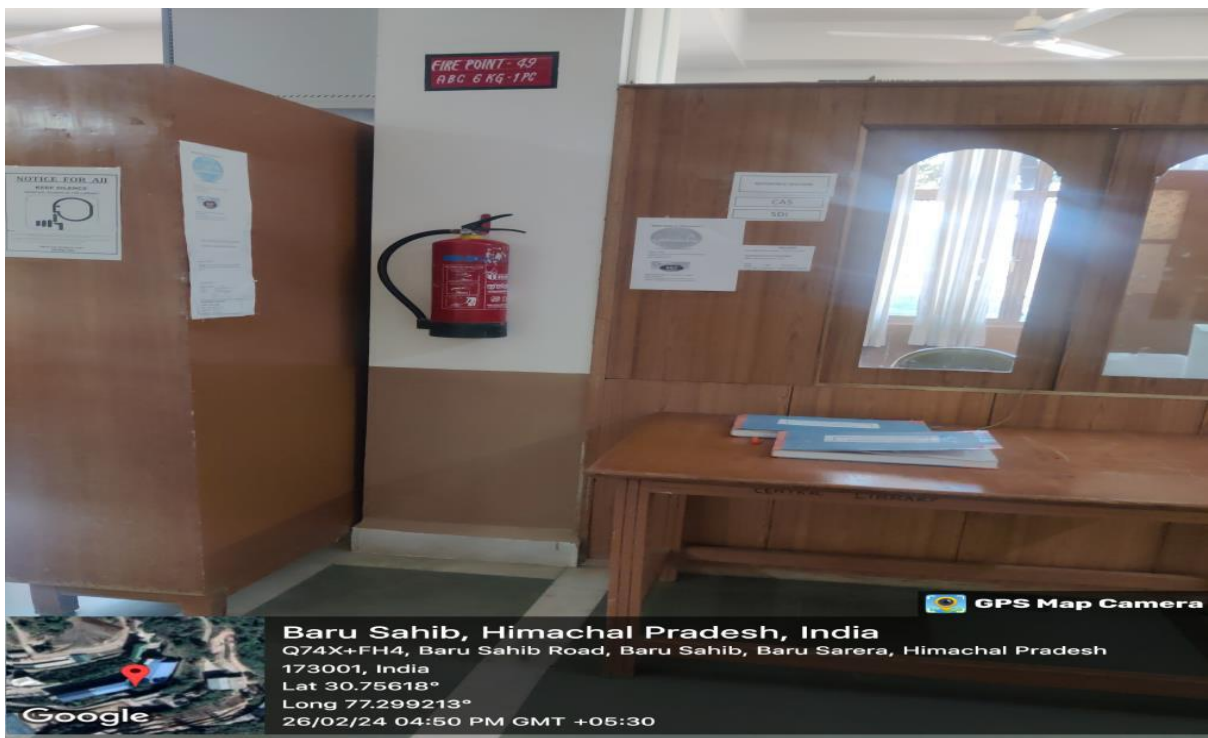
Fire Extinguisher Safety Measure
