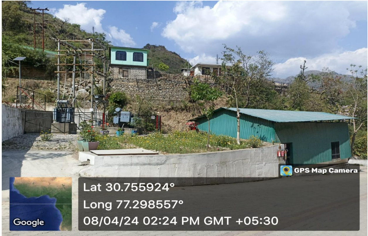
Transformer & Generator House
