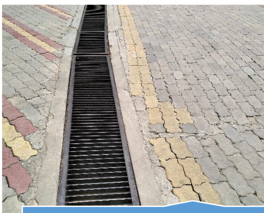
Storm Water Drainage
