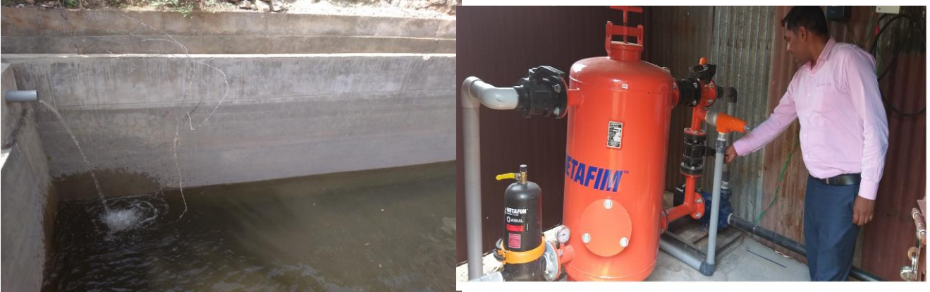
This photograph showing a water tank is constructed and linked it to electric pump with pre-filter
