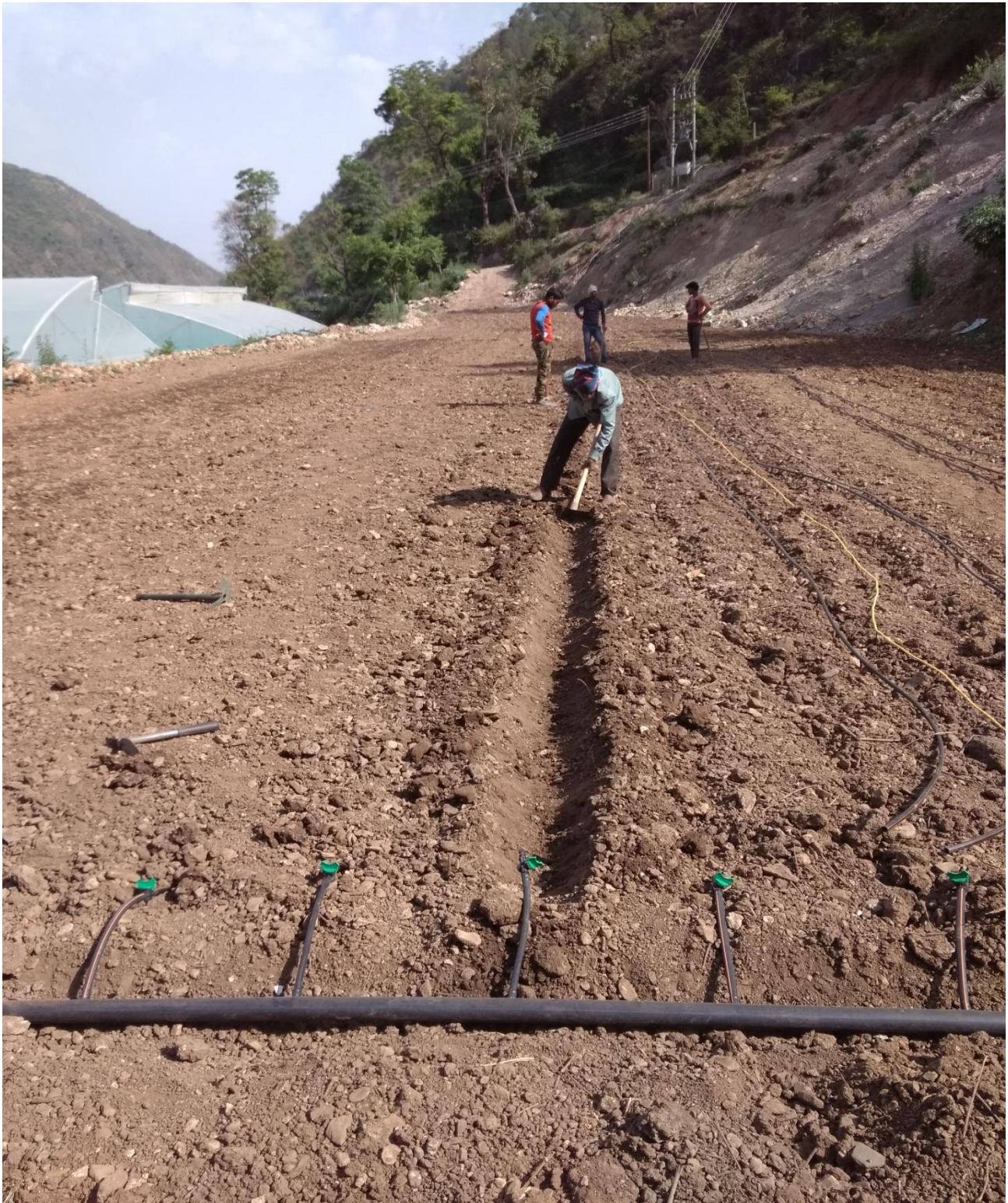
This photograph showing the labours are making optimum depth (15 cm) for installation of dripnet PC (lateral pipes)
