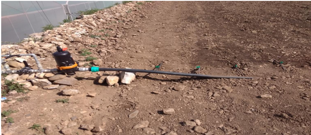
This photograph showing the installation of main line of subsurface drip irrigation with water filter, venturi injector and control valve
